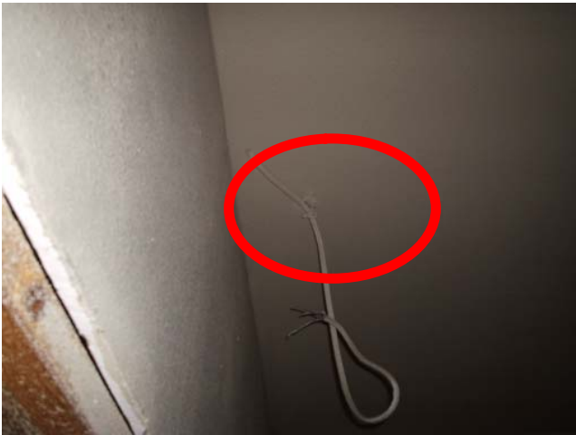
Light missing in laundry room
