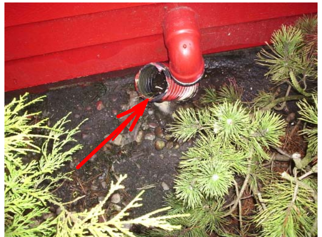
Down spout not connected to Leader, north side of building.
