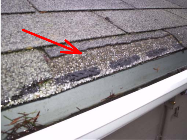
Damaged starter Shingles, back of house
