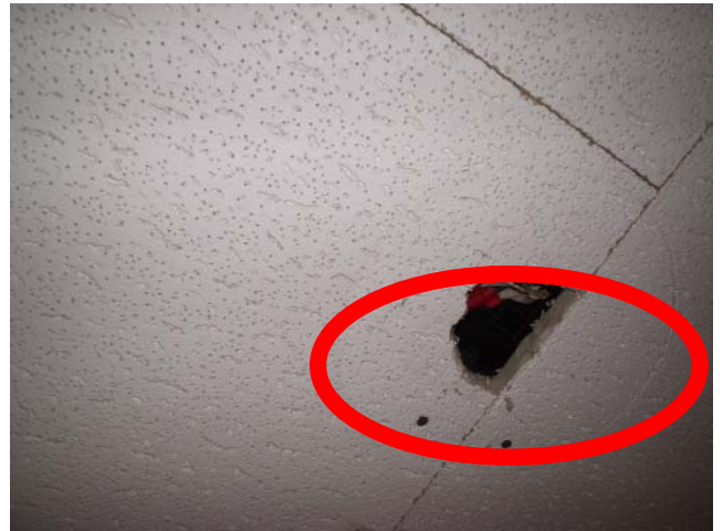
Missing cover on electrical junction box, Great Room
