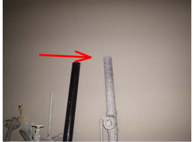
Washer Vent not plumbed thru roof.
